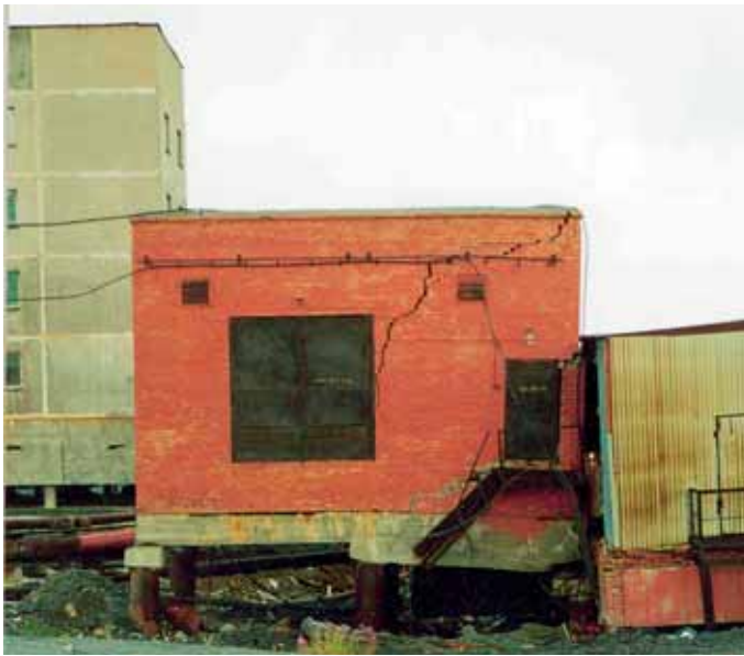
Fig. 2. Thawing of an ice-rich permafrost in the area of installation of underground utility line and resulting deformation of structure in the residential area of Oganer near Norilsk. July 2003
