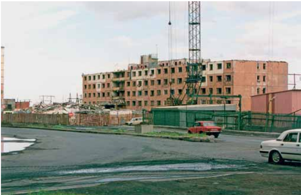
Fig. 3. Demolition of a nine-story residential building on Laureates St. in Norilsk after 21 years of operation, July 2001
