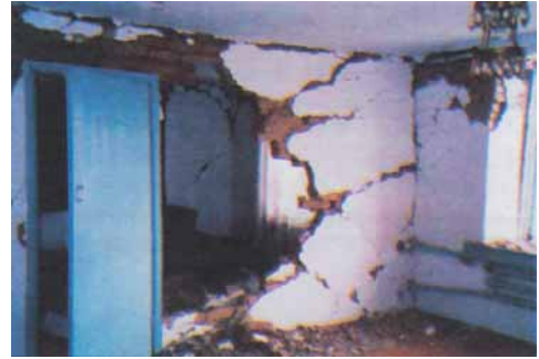
Fig. 11. Aftermath of the Lugovskoy earthquake in 2004.
