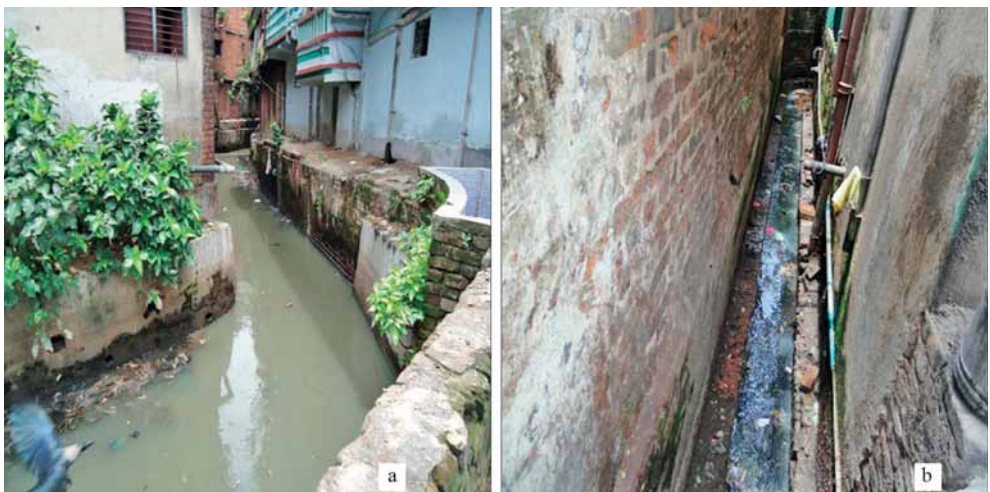
Fig. 4. Open drainage in Garden Reach, Kolkata.
